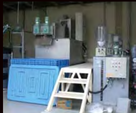
Excess Sludge at Industrial Plant (MDQ-202)
